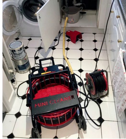
Photo courtesy of MT Drains
